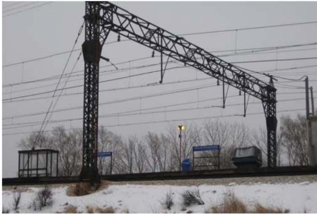
Figure 5-10: Metra Electric District Main Line Infrastructure and Track at 91st Street Station
