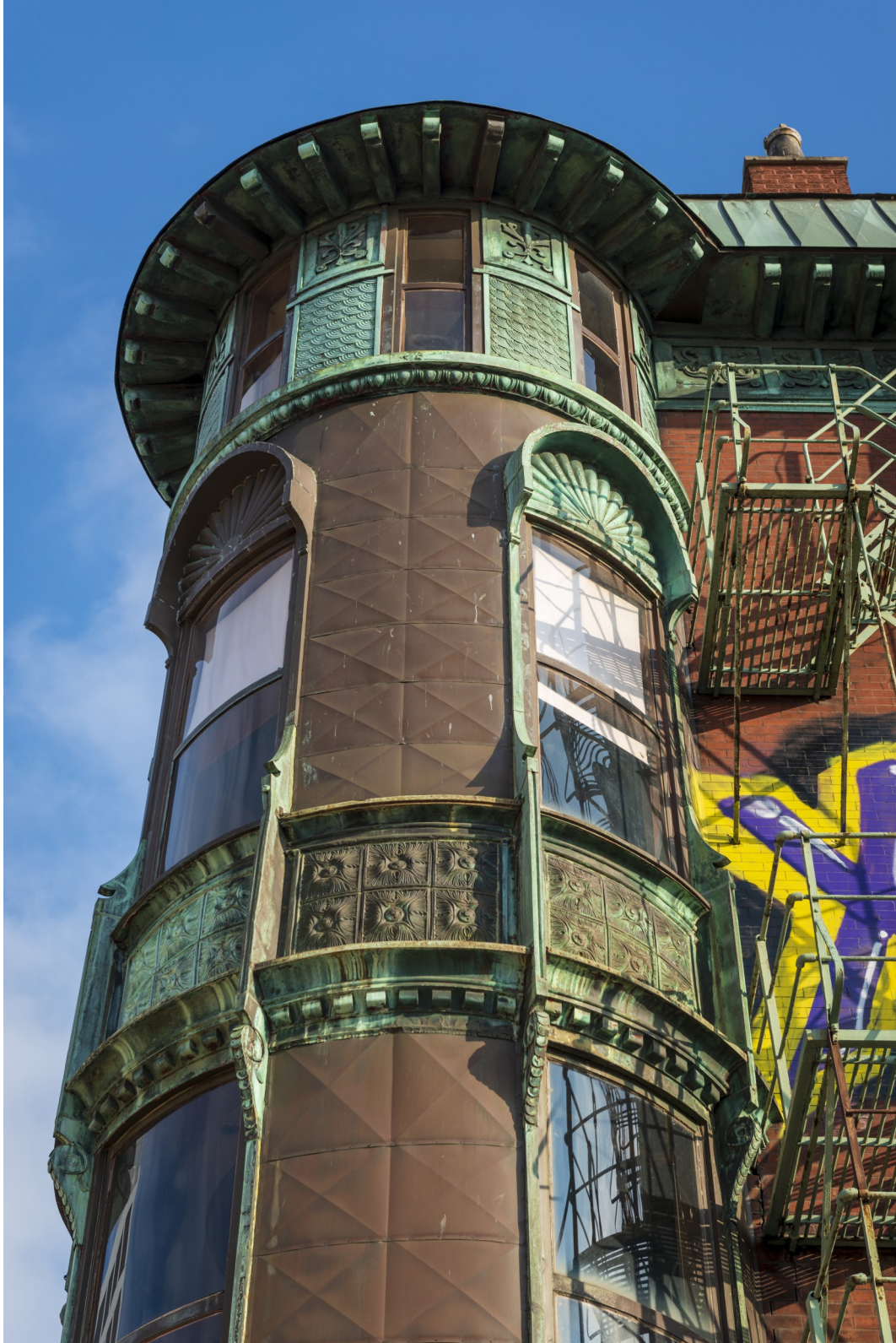
The corner turret of the (Former) Schlitz Brewery-Tied House, 1393-1399 West Lake Street. Replacement panels with a slightly raised "X" pattern are inserted at the second and third floors in between windows, leaving decorative spandrel panels, moldings, and window frames intact. At the third floor, portions of the window frame and the decorative fan lunette above were reproduced to match the existing. (Photo by Patrick L. Pyszka)
