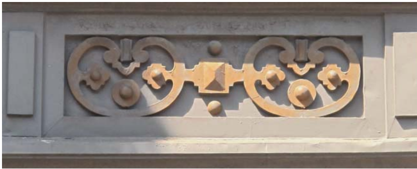
1944 N. Oakley Avenue displays several distinct features of the German Renaissance Revival style of architecture, including: the “bonnet” roof and semicircular lunette with shell-like fluting topping the bay (top), and the strapwork ornamentation (middle) at the base of the bay, all in pressed metal. The circa 1970 photo (bottom) shows the original gable roof above the bay, a German Renaissance Revival feature which no longer remains.
