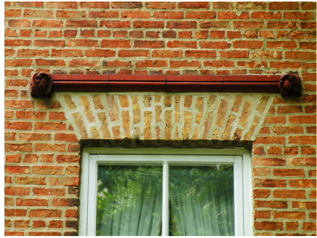
The later corner tower addition has flat arches with decorative red terra cotta drip moulds and foliate label ends. One larger terra cotta producer was the Northwestern Terra Cotta Company, which was founded in Chicago in 1878.
