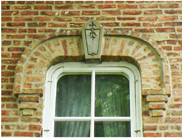
The original portion of the house features brick window hoods with cast stone keystones. Cast stone is a cementitious artificial stone that was widely produced in Chicago after it was patented by George A. Frear in 1868.
