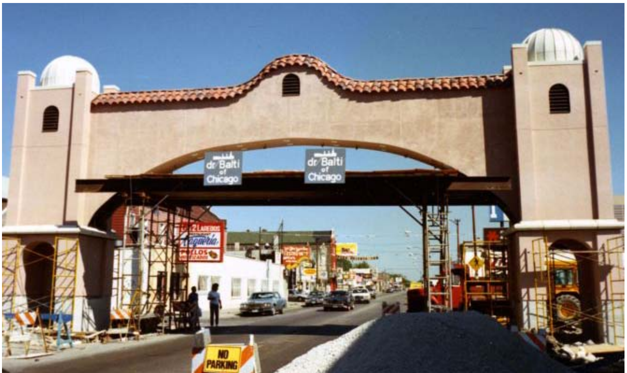
The arch across 26th Street in the Little Village neighborhood was built in 1990. Traffic was maintained during construction. Mortenson Roofing Company
