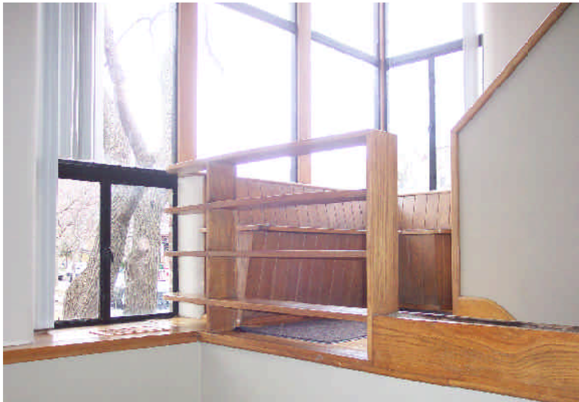
Top: A view looking down on the living room fireplace from the second-floor corridor, which connects two bedrooms and a bathroom. Bottom: A view from the living room looking up to the stairwell window wall and landing, with its built-in wood window seat.
