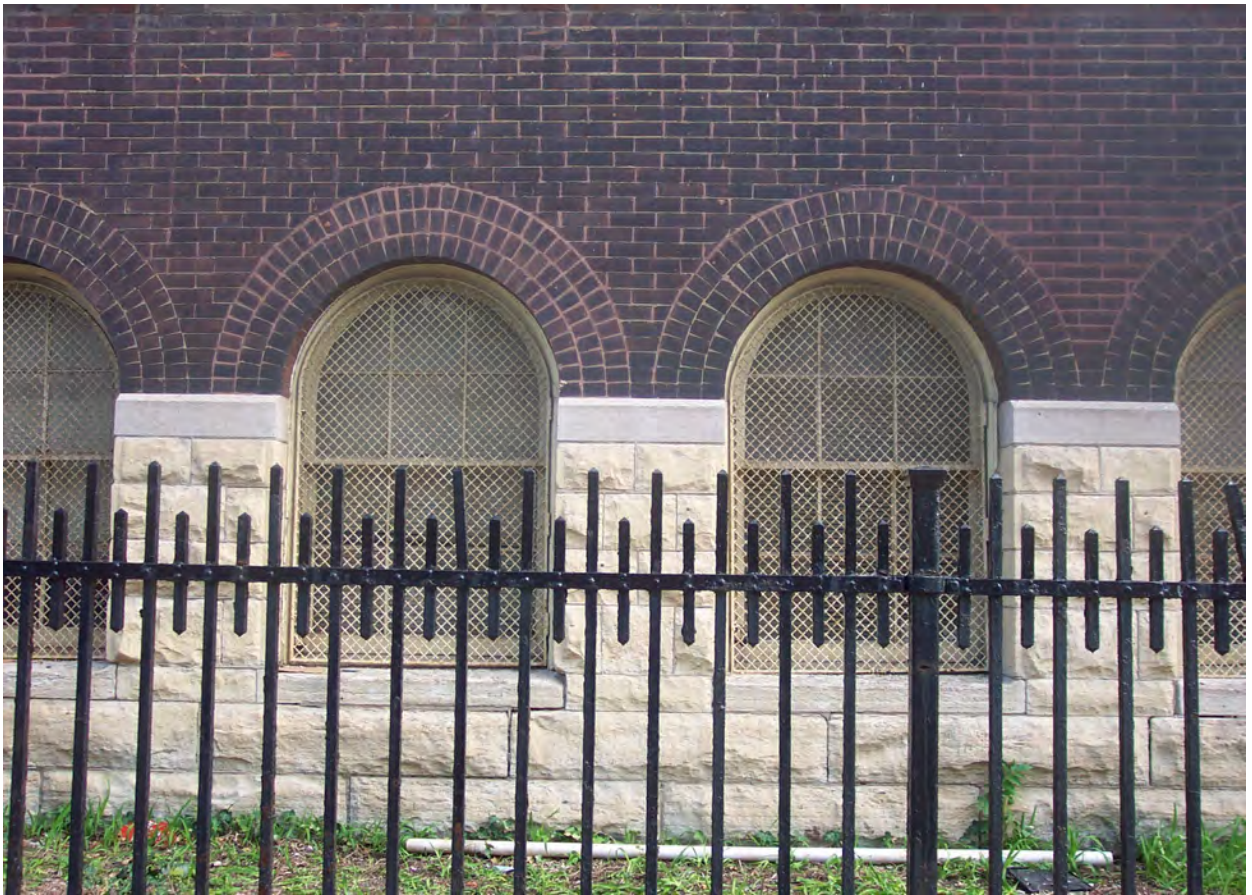
Views of the building's basement windows, ornamented with stone and brick, and the building's pressed metal cornice.
