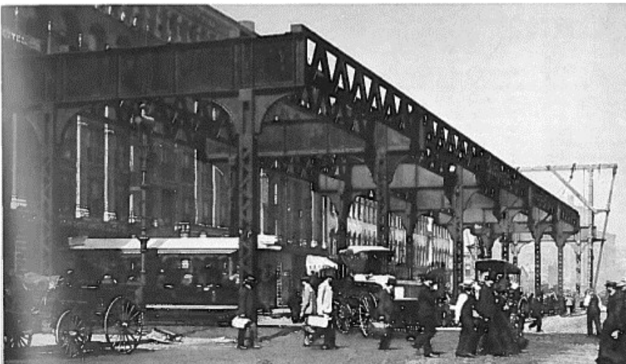
Before the Loop Elevated, the Lake Street 'L' originally terminated on Wacker Drive near Madison Street. Pictured is construction of the Lake Street Elevated Railroad on Wacker Drive. (Chicago Transit Authority Collection)
