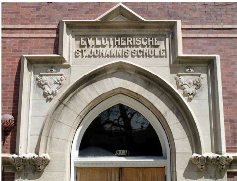
The German name of the school, Ev. Lutherische St. Johannis Schule , graphically conveys the building's former German ethnic identity.
