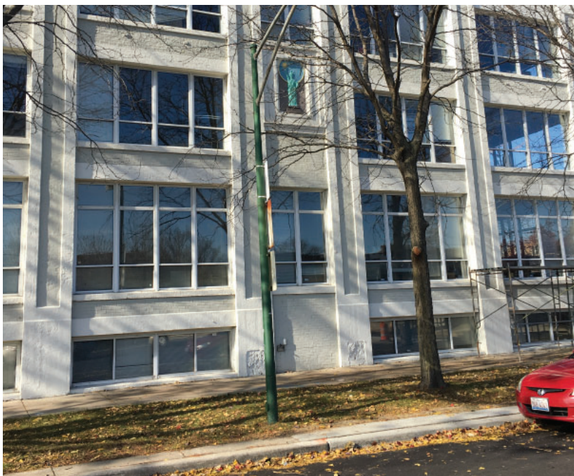
As an alternative to painting, staining stone architectural features can help preserve the masonry aesthetic and add color and contrast to buildings.
