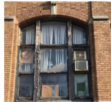
Retaining and restoring original wood and/or steel windows is encouraged. Replacement windows should be consistent in character and configuration to the original.
