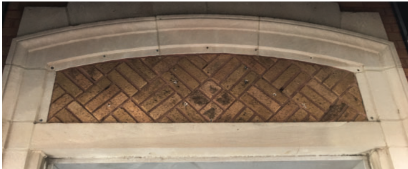
The combination of cast stone and brick inserts are also prevalent throughout Ravenswood industrial Corridor.
