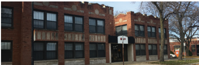
Window openings are typically consistent from floor to floor. Large storefront openings at the first floor are uncommon.
