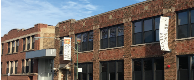
New signs should not obscure decorative building features and should be affixed without damaging the historic masonry.
