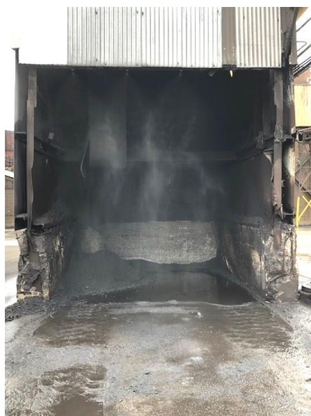
Figure 2 - "3-4 Junction" Building (showing water from overhead sprays)
