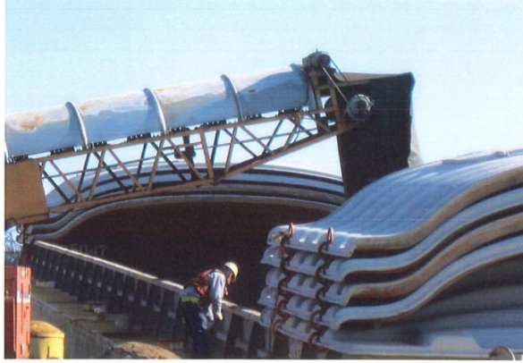
Figure 5 - Photo of Enclosed Conveyor with Chute Depositing Material in Barge
