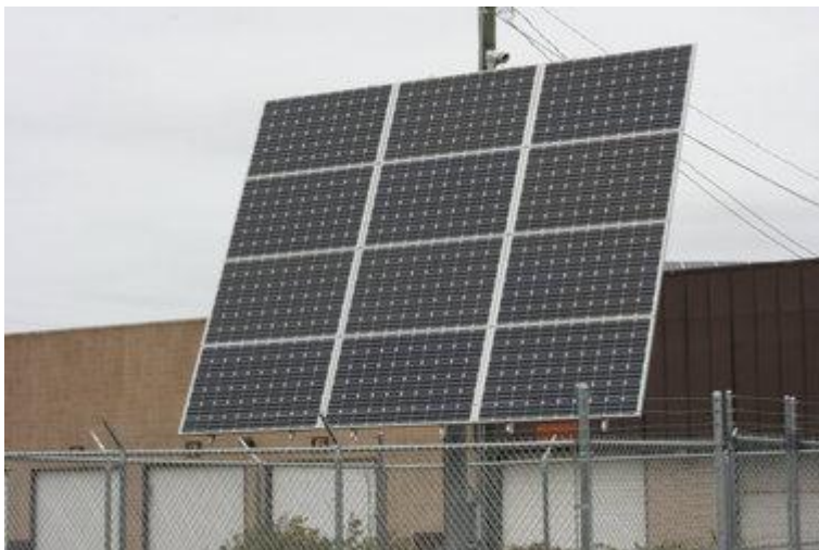
Figure 9: Single purpose pole-mounted solar PV system. (Source: http://www.mlive.com )
