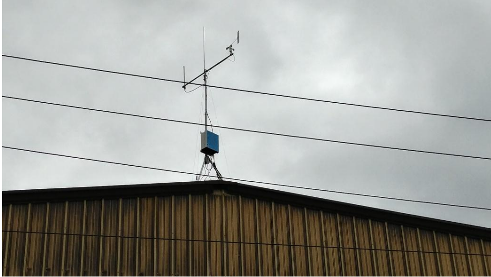
Image 1 - Picture of Weather Station (installed)
