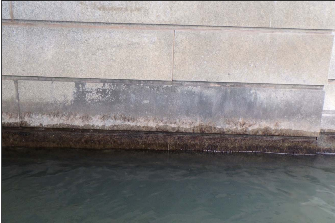
Photographs 3: View of the Typical Masonry Condition at the Waterline of the North River Pier, Looking North.
