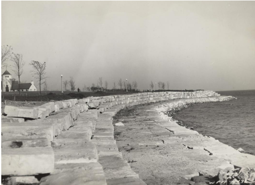
Figure 6. Construction of step-stone revetments on southeast side of Promontory Point, ca. 1938, Chicago Park District Records: Photographs, Chicago Public Library Special Collections.
