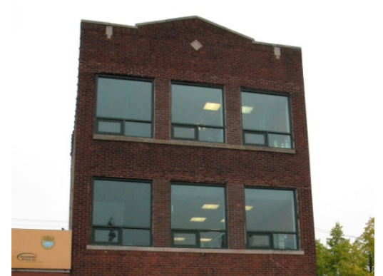
Inappropriately proportioned windows
