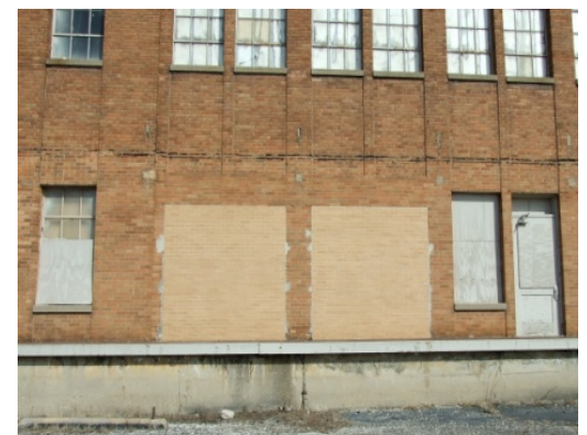
Inappropriate treatment - do not brick in door openings
