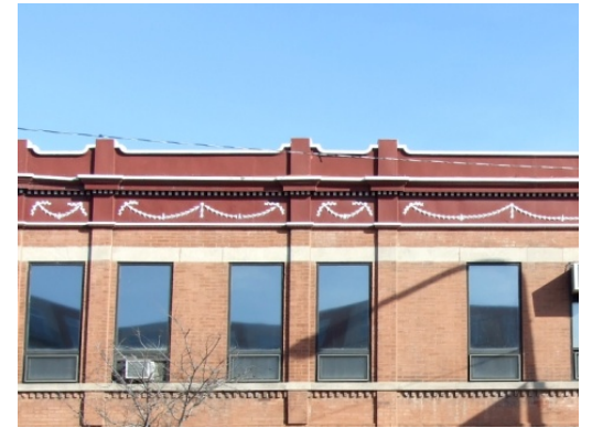
Inappropriately proportioned, mirror glass windows
