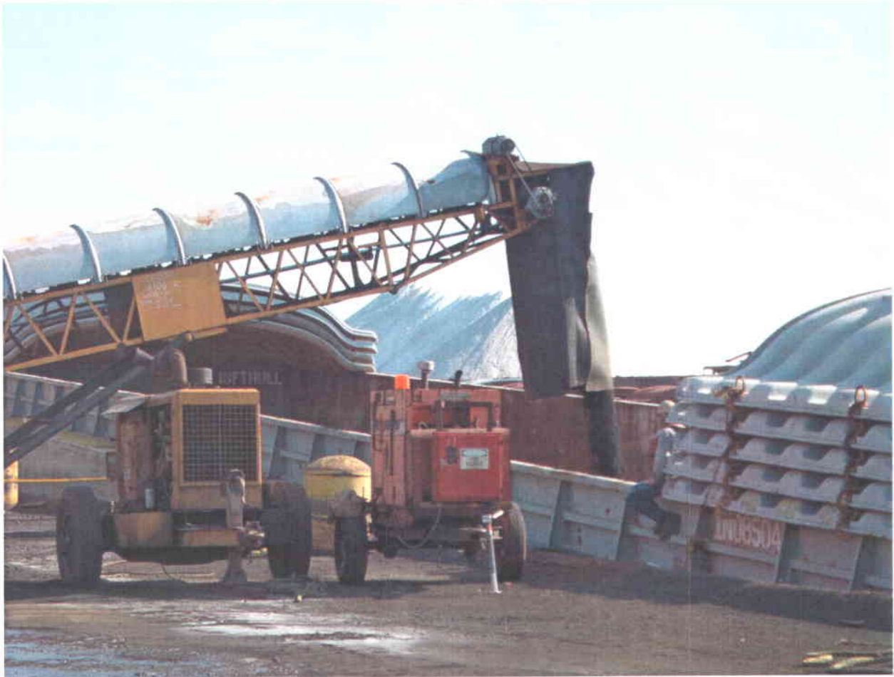
Test 1B – Barge Loading Covered Conveyor System
